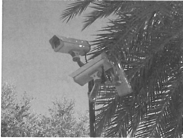
Typical security camera
