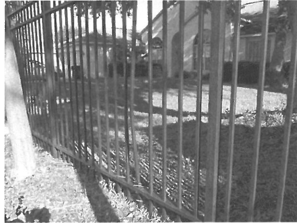
Damaged aluminum fence at entrance
