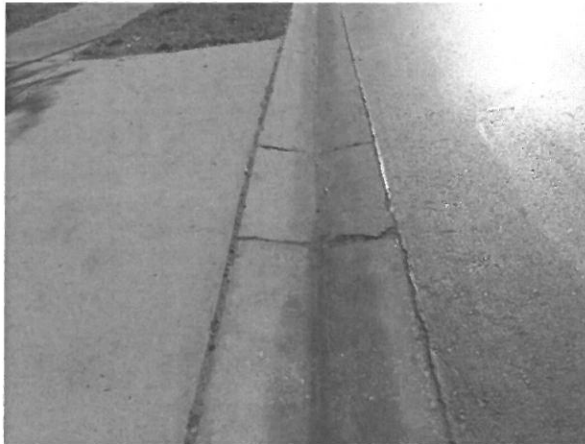
Typical concrete gutter. Note cracked gutter.
