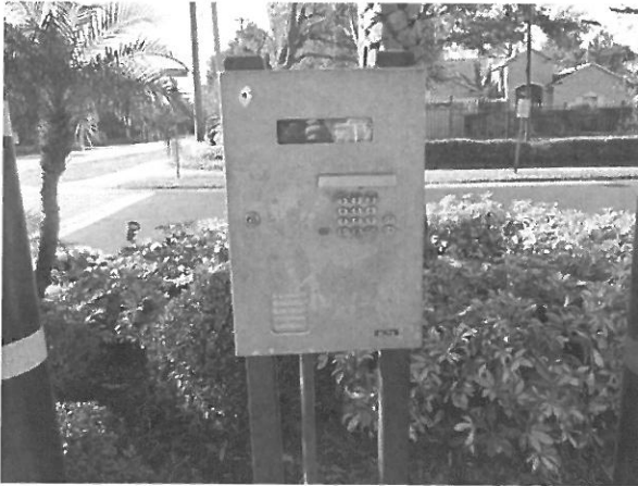
Gate entry panel
