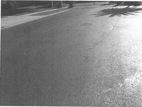
Asphalt pavement at Reagan Trail with patch and longitudinal cracks
