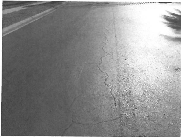
Asphalt pavement at Reagan Trail with longitudinal cracks
