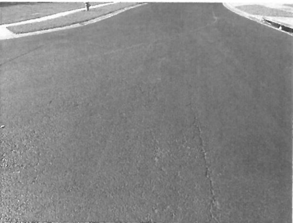
Asphalt pavement at Reagan Trail with cracks
